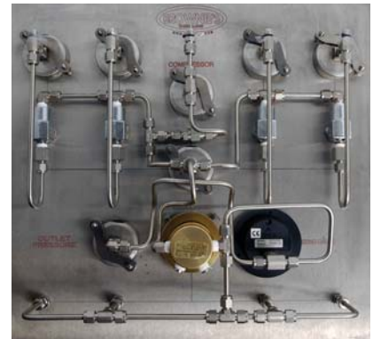
Panels for Brownie’s tankfill systems feature a variety of stainless steel Swagelok components.
